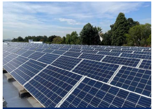
Solar PV panels at Adcorp Place.
